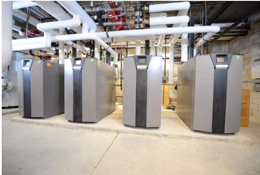
Traditional Heating System
